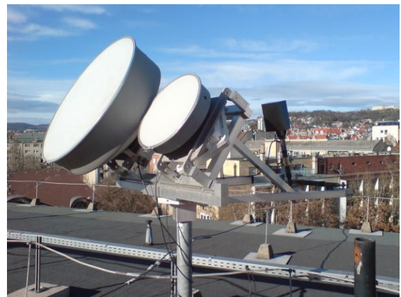
Fig. 2. High performance antennas and the tracking system
