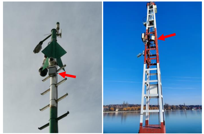
Fig. 6. Unit installations at the entry posts of the marinas.
