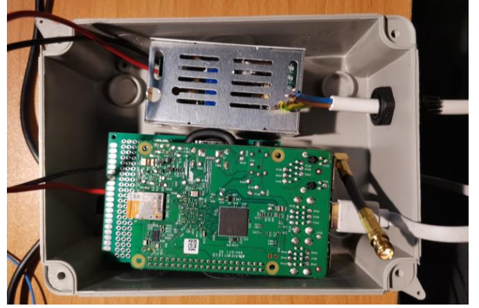
Fig. 3. Inside the enclosure of the measurement unit (without antennas).
